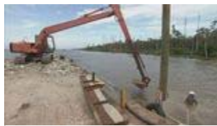
A crew deposits rock rubble along an area of Mobile Bay shoreline near Weeks Bay
